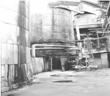
Figure 23.1. Leakages at a production plant
