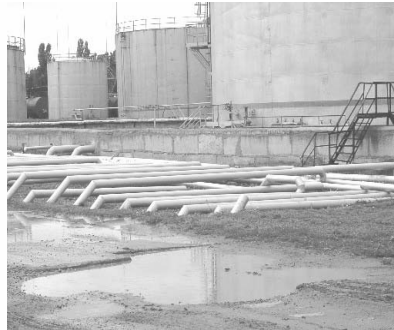
Figure 23.2. Single wall pipe subways through retention room; no knock-down protection
