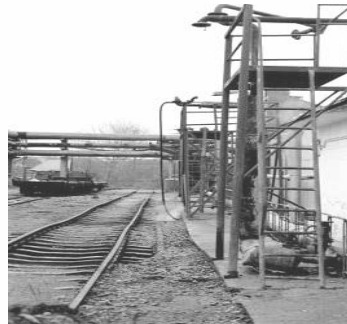
Figure 23.4. Unloading station for hazardous fluids from railroad tank cars
